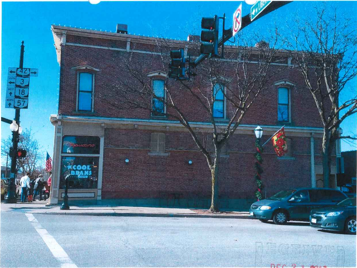
East Face (N Court St)
