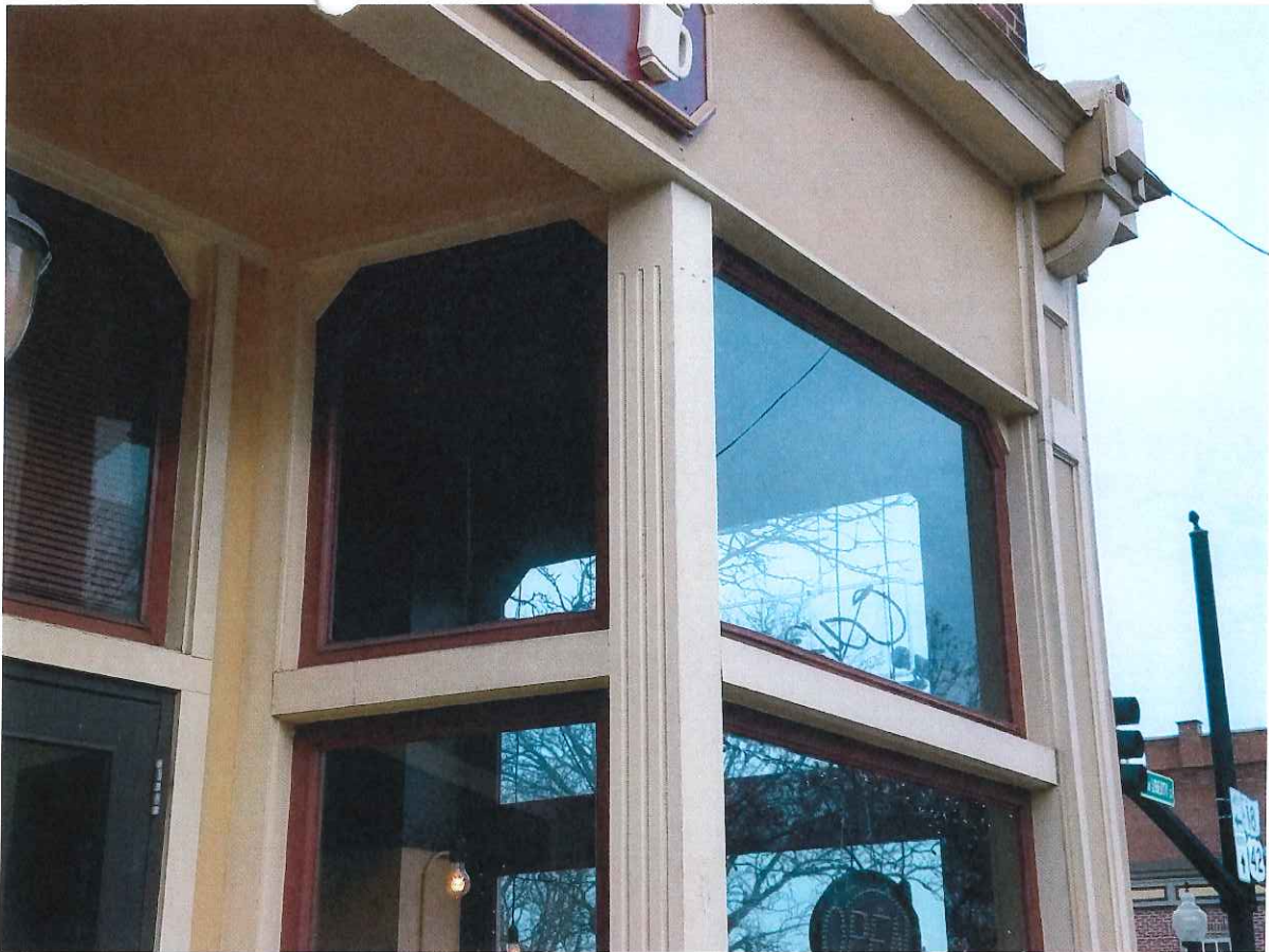
South Face (W Liberty St) First Floor Upper Windows Right of Cool Beans Entry Upper right window only being replaced.
