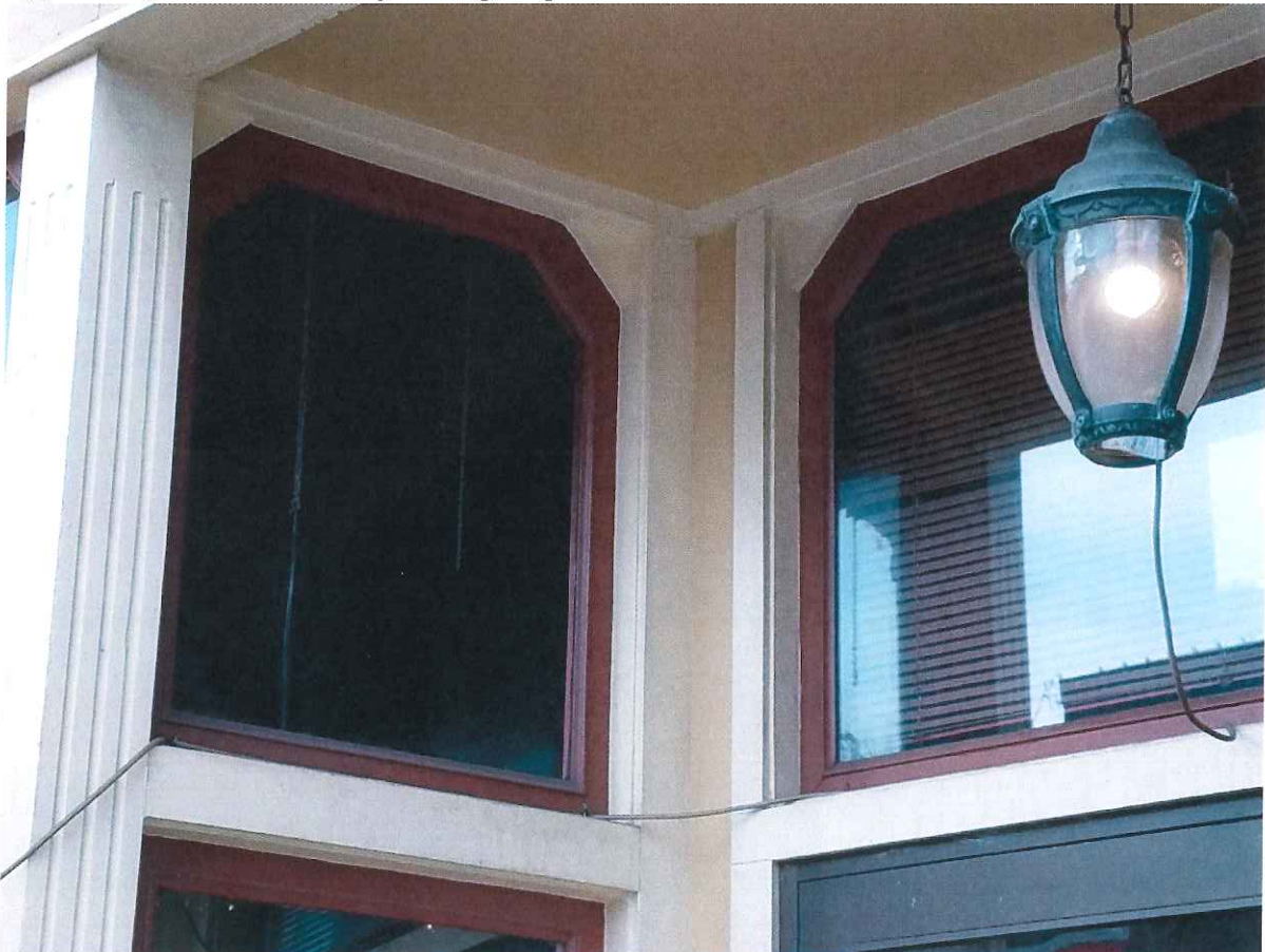
South Face (W Liberty St) First Floor Upper Window Left of Cool Beans Entry
