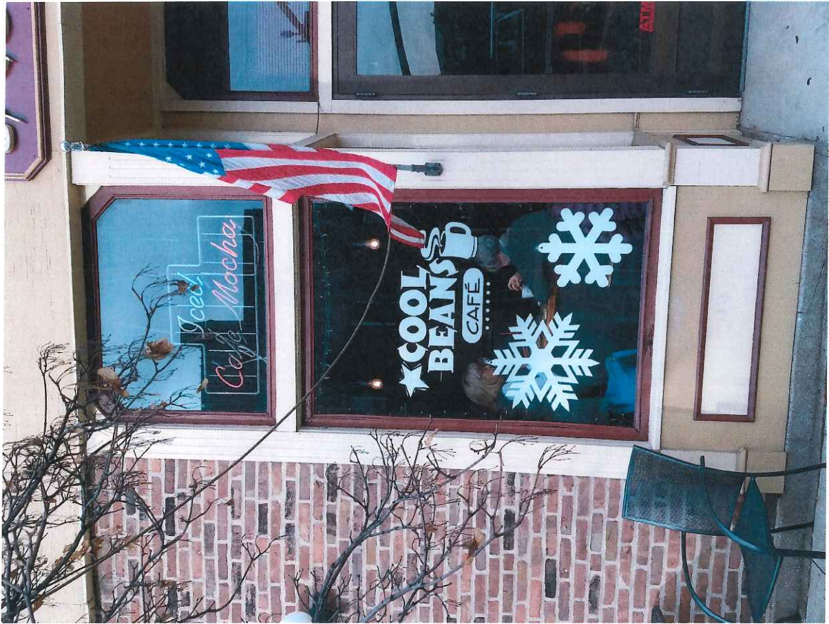
South Face (W Liberty St) First Floor Windows Left of Cool Beans Entry
