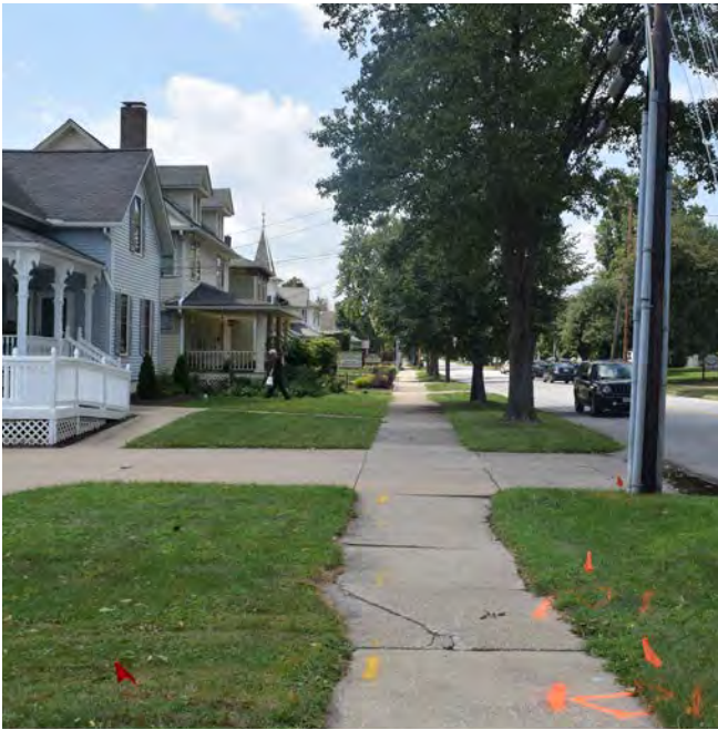
Typical sidewalk condition along West Liberty Street.
